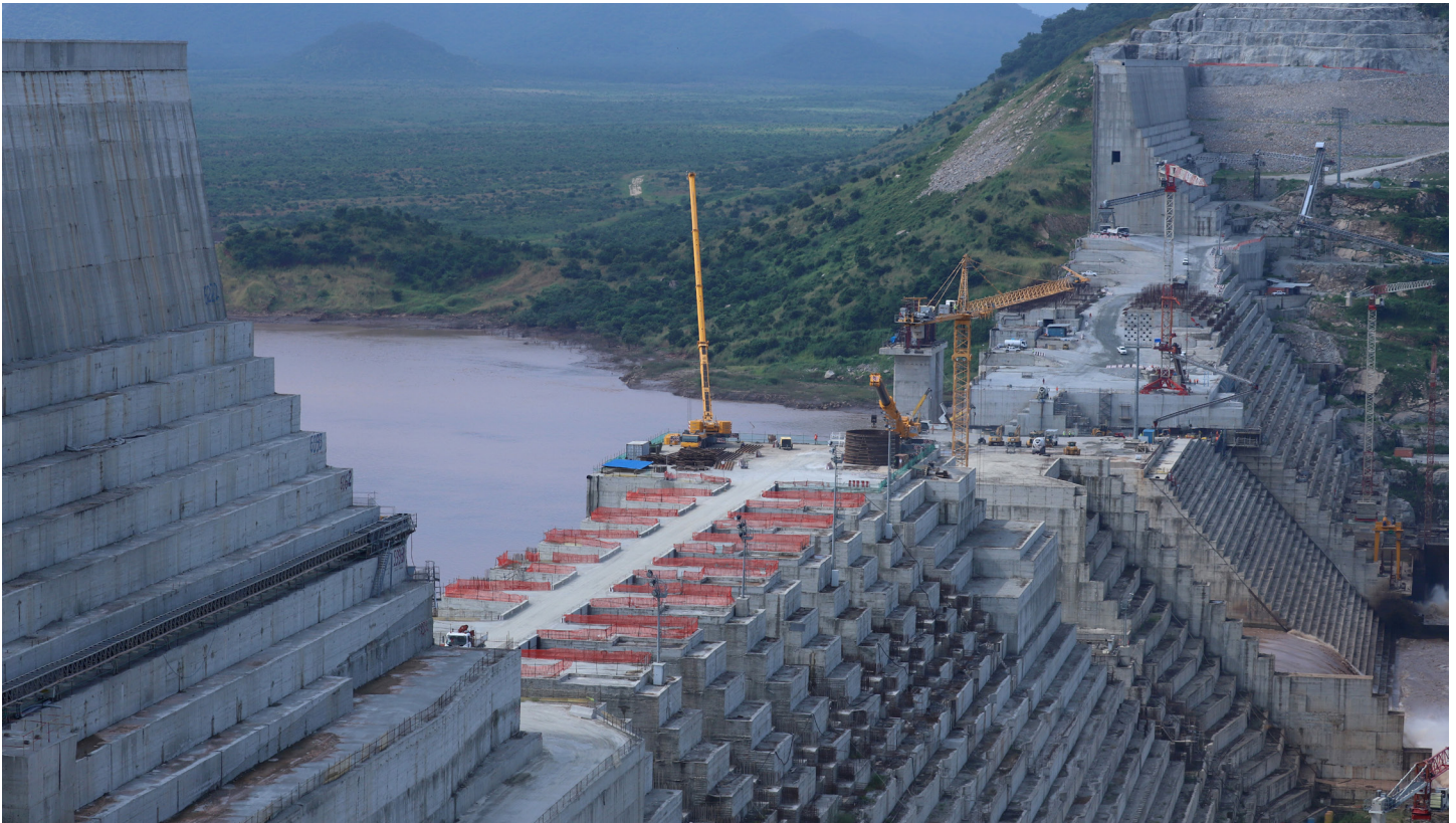
Ethiopia's Grand Renaissance Dam is seen as it undergoes construction work on the river Nile in Ethiopia on September 26, 2019. Source: REUTERS/Tiksa Negeri
